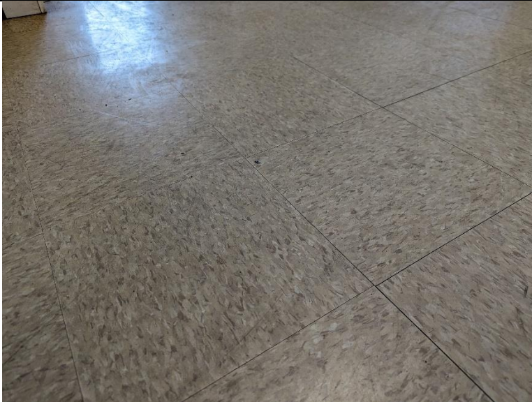
19) Vinyl Floor Tile – Hallway – Vinyl Tile(5% Chrysotile) underneath these tiles is ACM
