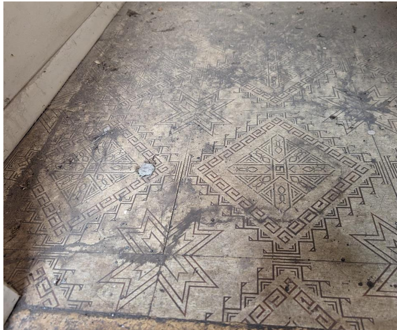
Photo ID #'s 18,19 – Patterned Vinyl Floor Tile found in the Workshop Bathroom as well as underneath Vinyl Floor Tile in the Hallway.
