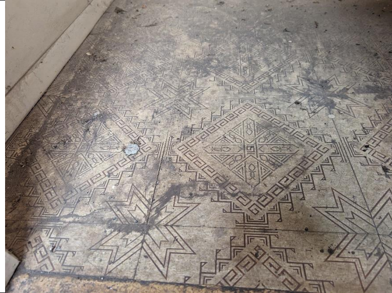
18) Vinyl Floor Tile(5% Chrysotile) – Workshop Bathroom
