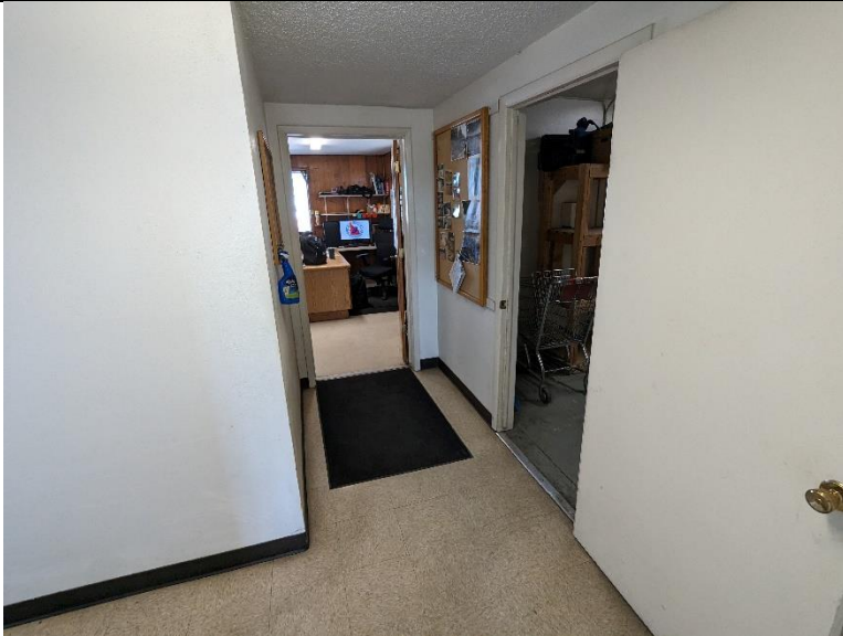
7) Hallway – Vinyl Tile(5% Chrysotile) found underneath visible tile is ACM
