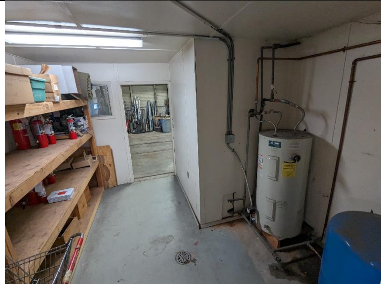
12) Water Heater Room
