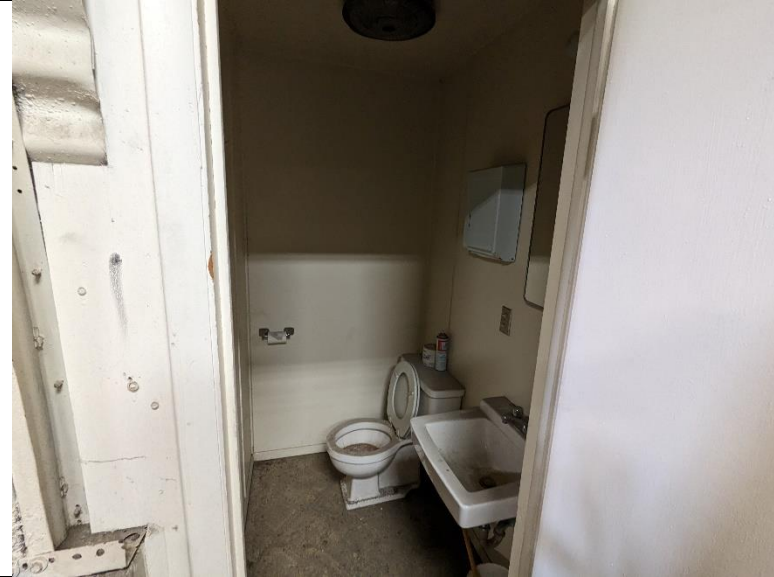
14) Workshop Bathroom – Vinyl Floor Tile(5% Chrysotile)
