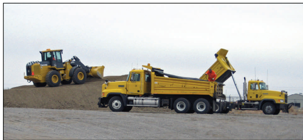
Shoshone Maintenance works on the pile of fill for the new District 4 Headquarters west of the current administration building in Shoshone.
