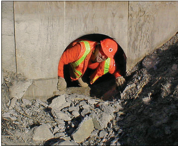
Peek-a-boo ... Finding the easiest way through a new culvert on Idaho 24 was Rupert's newest mole, Travis Morrell. (Picture by Warren Kell)
