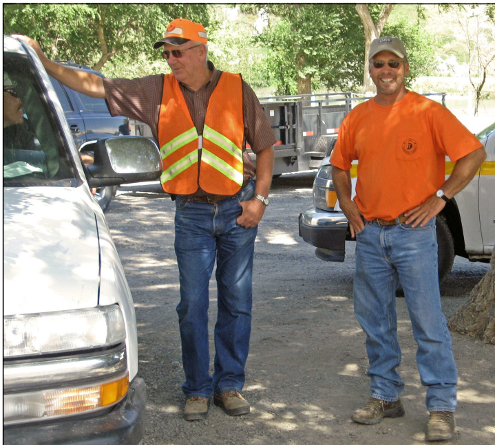
Never let anybody tell you these guys are true professionals. Ken Brott and Ken Lively found the best place to be on a hot day while still watching the construction zone.
