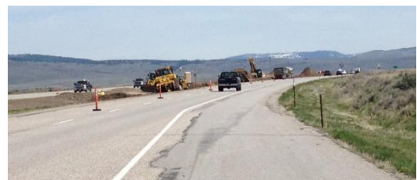
Crossovers will allow all traffic to use southbound I-15 while the northbound lanes are resurfaced.
