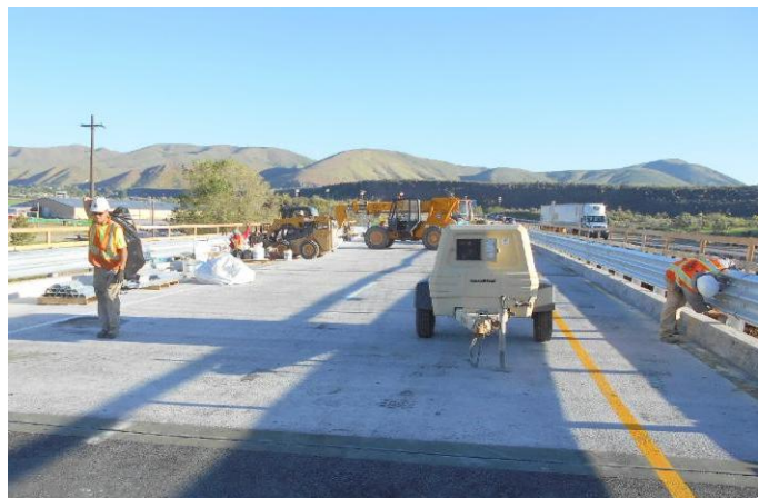
Work on the southbound Portneuf Bridge near Inkom is complete. Crews will move to the northbound Portneuf Bridge in early June.
