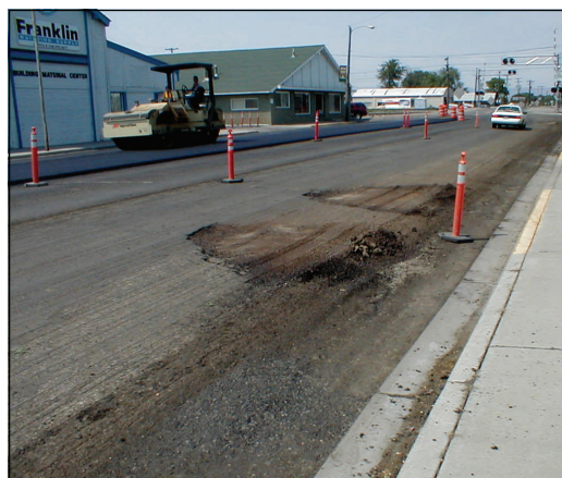
Paving on Idaho 46 through Gooding took place in mid-July and is now completed.
