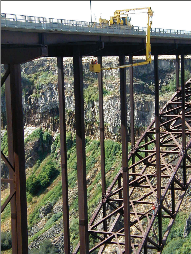
Above: The bridge inspection crew from Boise dangles both from above and on the narrow cross beams below to inspect the Perrine Bridge on July 17
